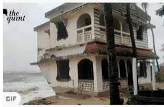
Cyclone Tauktae: House Collapses ... thequint.com
